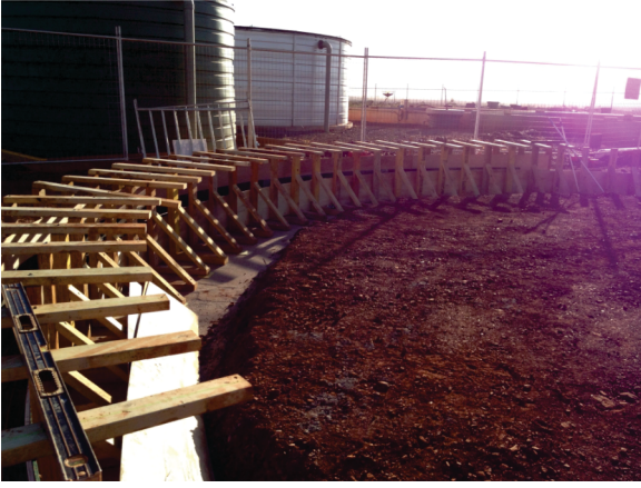
West Angelas, Waste Water Services Ring beam for waste water treatment tank
